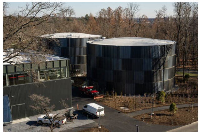
The system’s water tanks, one for hot water, the other cold, each hold 2.2 million gallons. Credit...Maansi Srivastava/The New York Times
