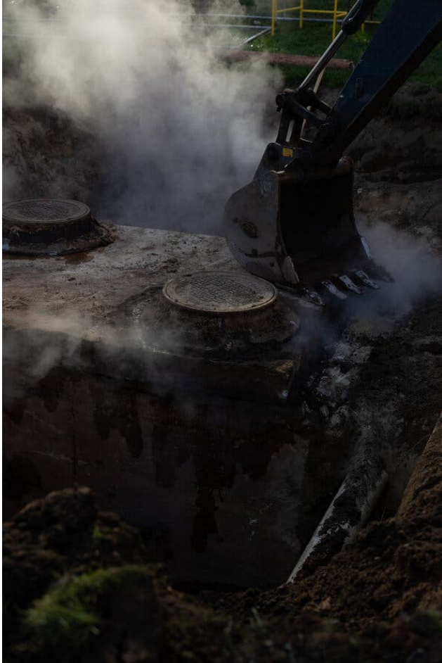
An old steam system site being deconstructed to make room for a geexchange well. Credit...Maansi Srivastava/The New York Times
