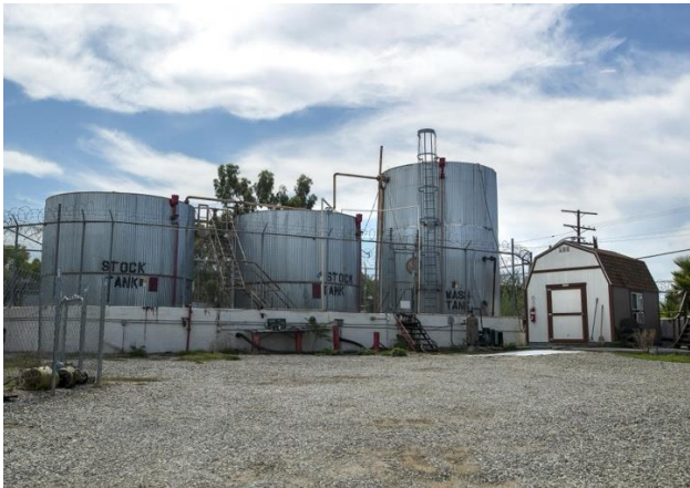
Storage tanks holding oil and other chemicals sit next to an active oil field in Westlake. (Mel Melcon / Los Angeles Times)
